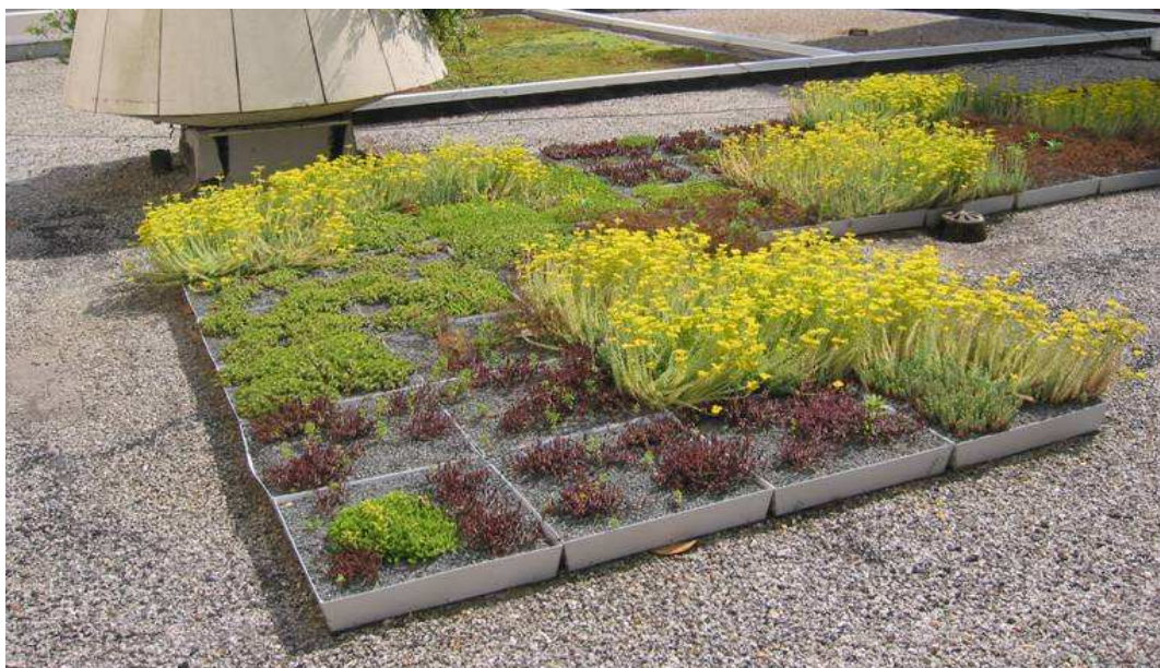
Figure 2. UGA modular green roof system.
