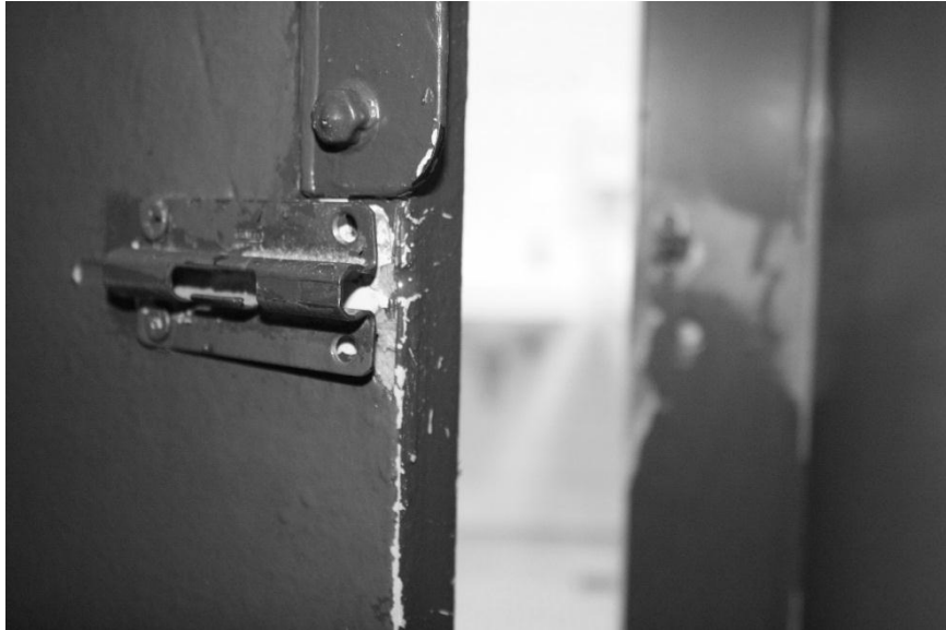
Figure 10. Broken bathroom door.
