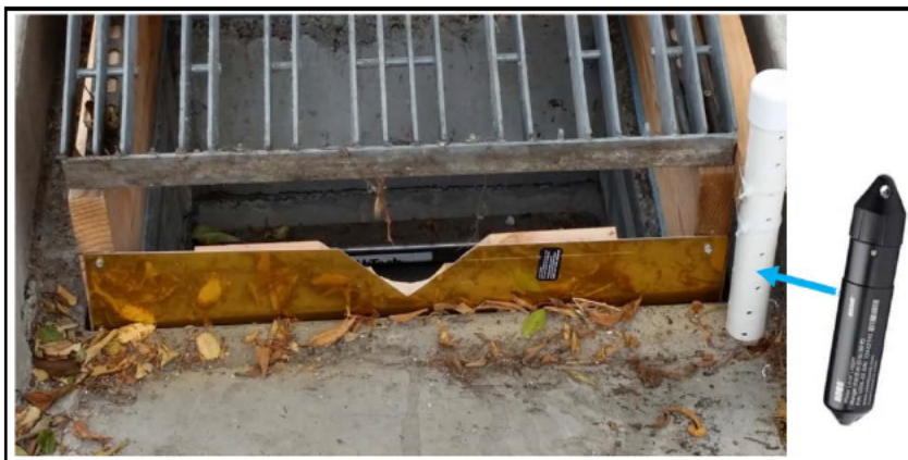
Figure 4. V-Notch weir in position at Inlet No. 3. The inset shows the HOBO data logger that rests at the bottom of the perforated PVC pipe attached to the weir.
